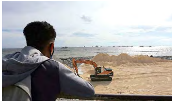
BAY WATCH A man watches as a construction worker spreads dolomite sand in Manila Bay. The bay’s beautification drew criticism and stirred debates. PHOTO BY ENRIQUE AGCAOILI
